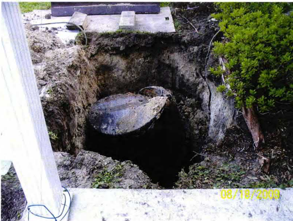
Picture 2: UST 1172Bobwhite.
